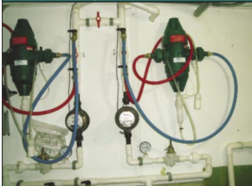
Figure 3. Newly Constructed Wean-to-Finish Facility with Medicators Connected to Waterlines with 1/2-in. Washing Machine Hoses
